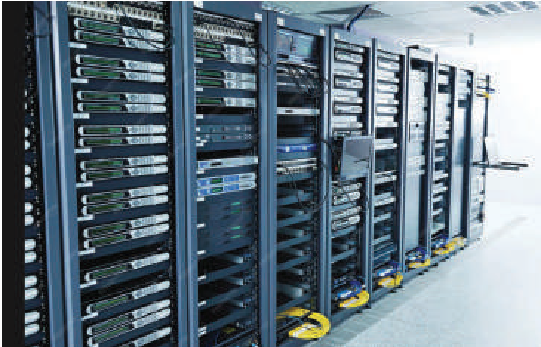
A server room
