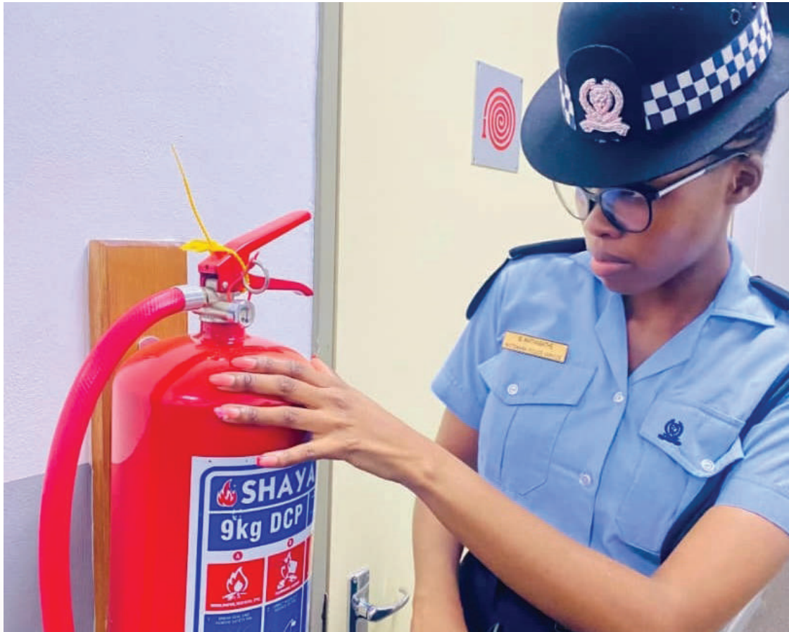
A SHE officer inspecting a fire extinguisher
